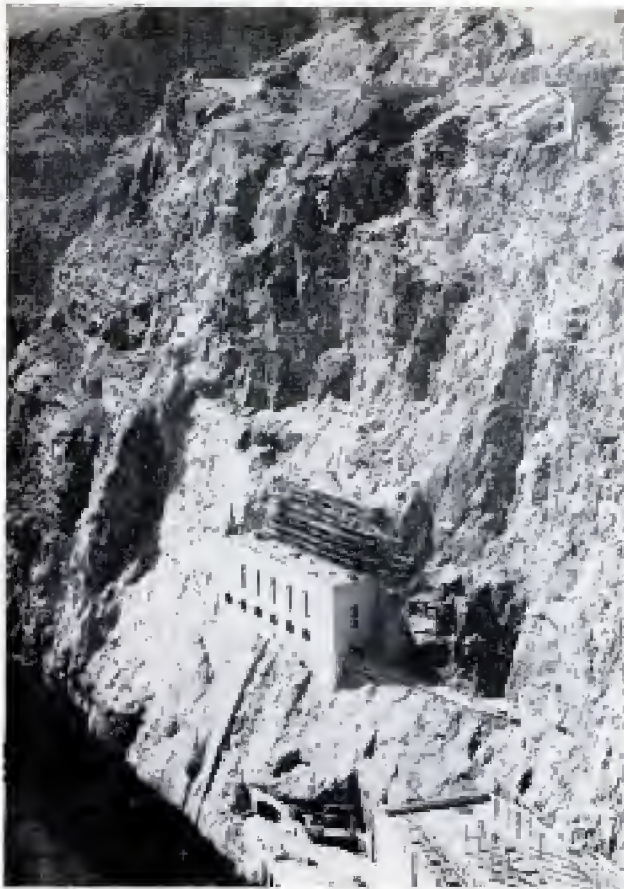
Huge rock slab hangs just above the valve house. Scaffold for the workmen was built around the slab
